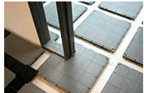
Full height partition erected on top, by fastening floor track to the UniPanel.
