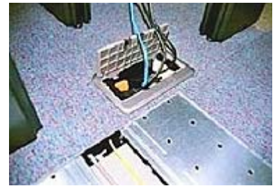
Extension and connection from Cable Trenches through service box SB-603
