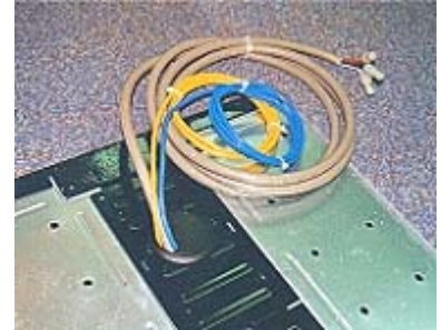
Cables extending from Cable Trenches to workstations or partition
