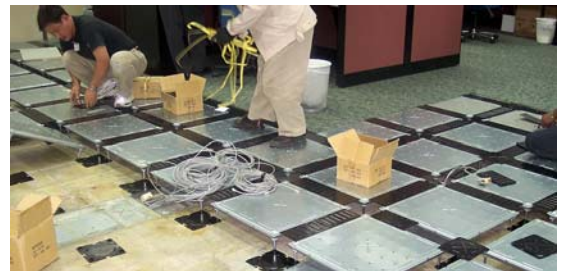
Camass installed on top of old embed floor trunks- Renovation in one room, other rooms working
